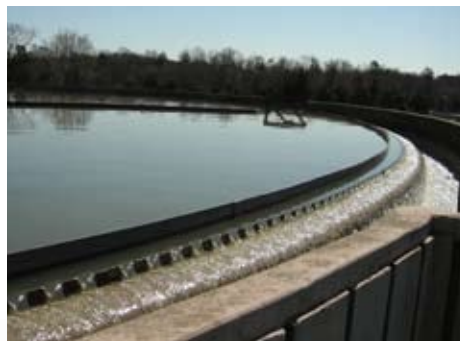
Wastewater clarification unit for reclaimed water production
