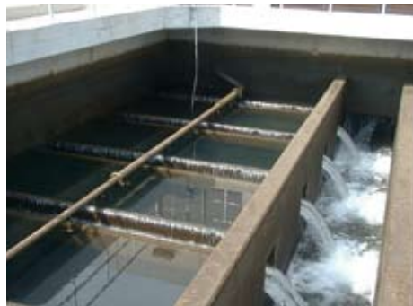
Backwashing of a filter at a water treatment plant
